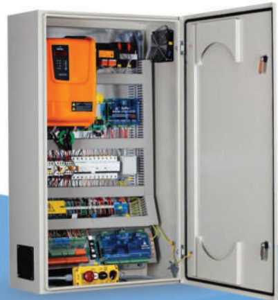
Integrated Control Panel
