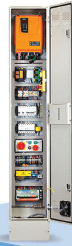
MRL Control Panel
